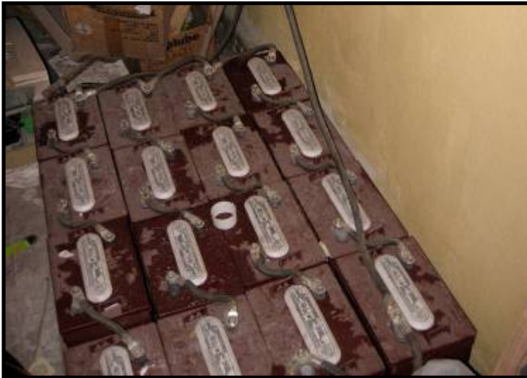
Figure 1: The batteries on the blood bank's UPS system have failed.
