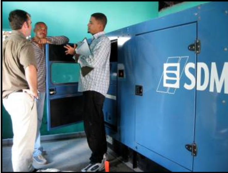
Figure 2: Although operational since 2006, no preventative maintenance has been performed on the hospital's generator.
