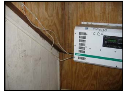
Figure 4: Small gauge wire is both a fire hazard and prevents proper operation of the inverter.
