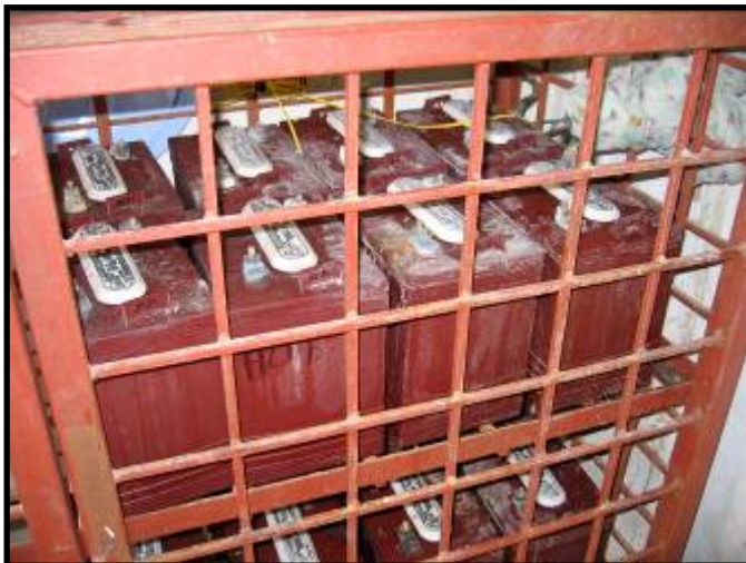
Figure 4: The PEPFAR provided inverter was not functioning because the battery cables had been stolen. Smaller mesh on the battery cage would deter future theft.
