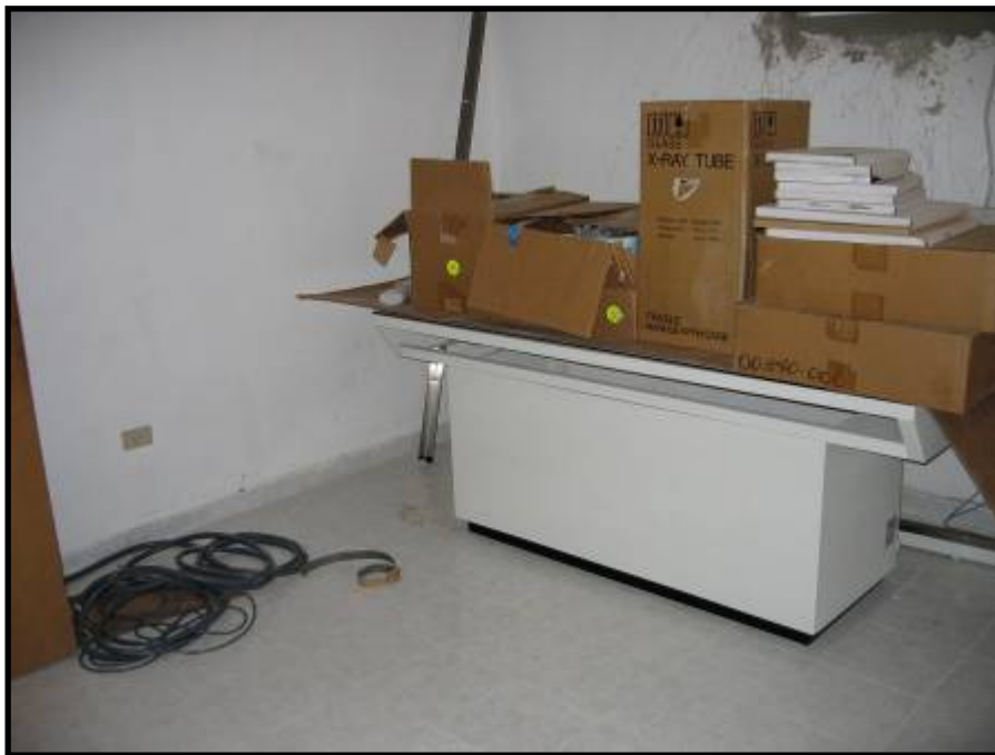
Figure 2: X-ray machine not installed because of insufficient power supply.
