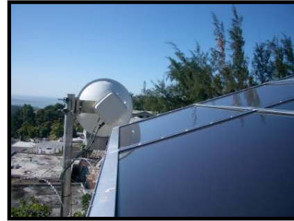
Figure 3: Special solar array mounts prevent individual panels from being removed, greatly deterring theft.
