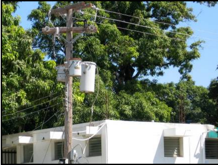
Figure 1: Three-phase transformers inoperable
