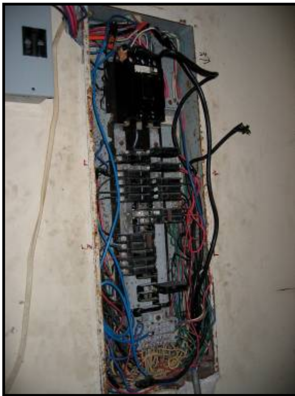
Figure 2: Poor wiring which is typical of many clinics in Haiti.
