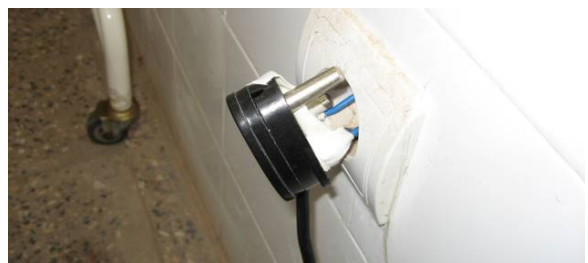
The pins on this autoclave plug have been taped so staff can try to use it in an inappropriate outlet.
