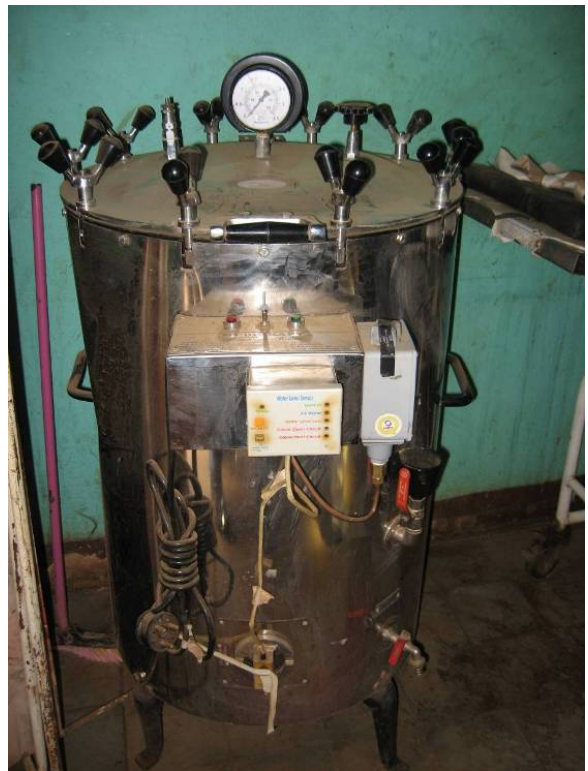
A new sterilizer unable to be used because the health center lacks the proper wiring.
