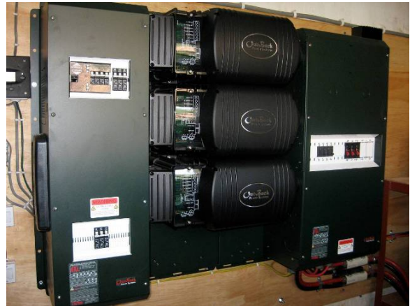
Inverters at a health center in Rwanda.
