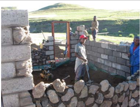
Sometimes the buildings are not quite Ready when we get there.
