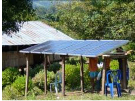
Solar Panels at DPN Hospital
