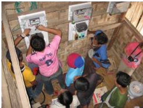
Medics work on the charge controllers and inverters in the equipment room
